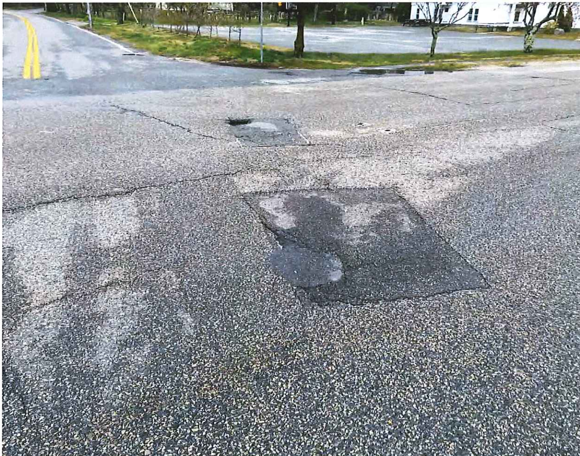
Pavement patch deterioration
