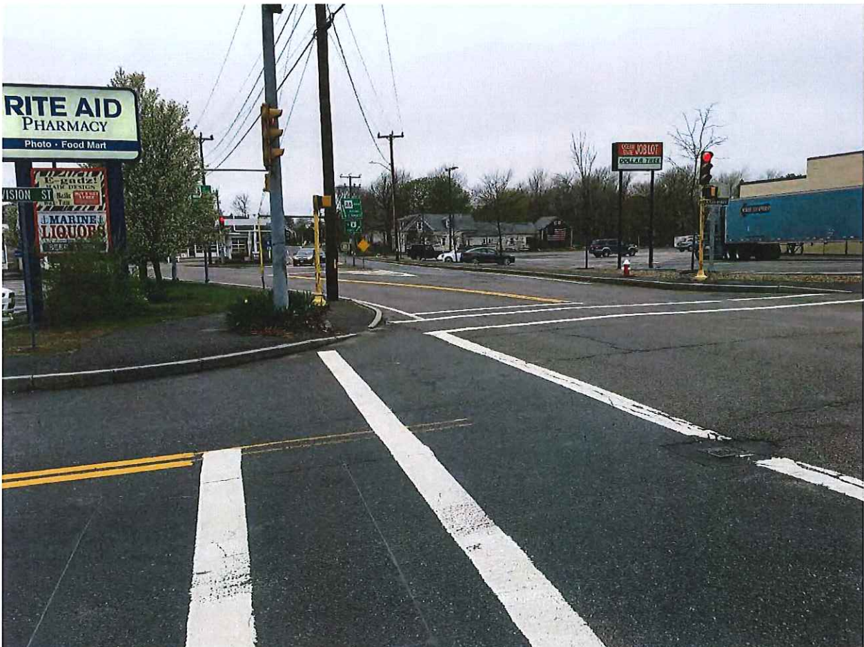
Lack of ADA/AAB compliant curb ramps and pedestrian activated traffic equipment at Division Street intersection
