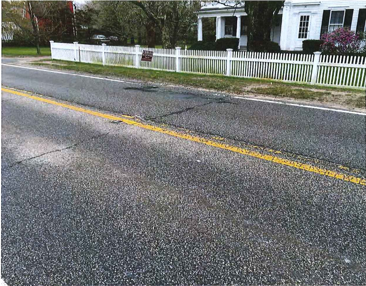
Faded pavement markings
