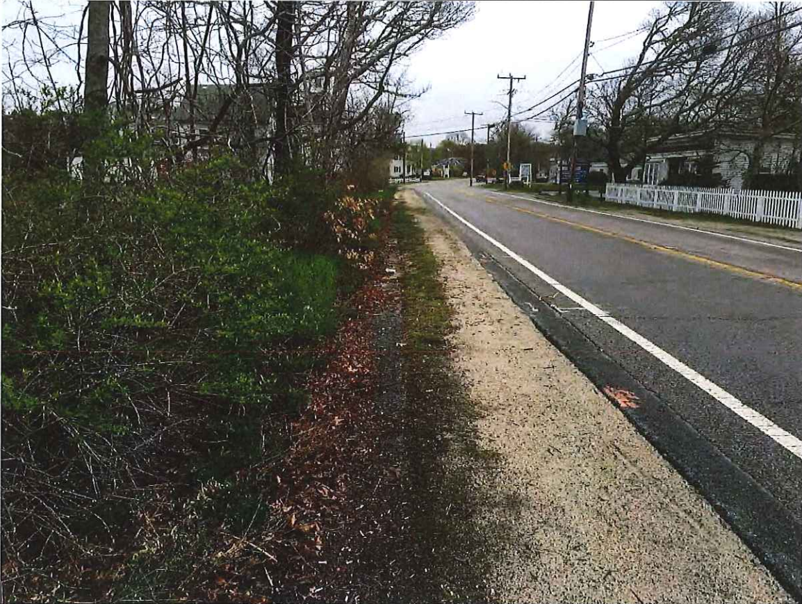
Poor condition of sidewalk along the northern side of Route 28
