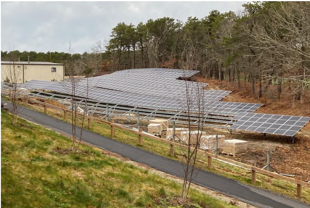
Completed Stand Alone Field: Total Project Generation 282KW
