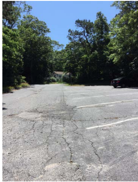
Photo Caption: Looking uphill at upper portion of parking lot – note the condition of the pavement.
