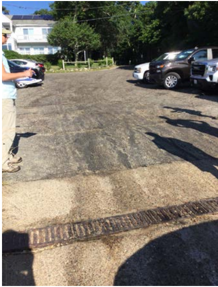
Photo Caption: Clogged trench drain at boat ramp
