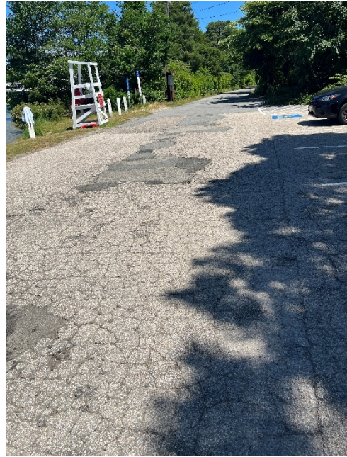
Photo Caption: Parking lot in need of improvement
