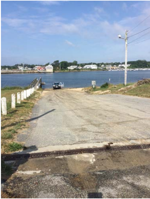
Photo Caption: Boat ramp with dock on the left and the clogged trench drain in the foreground.
