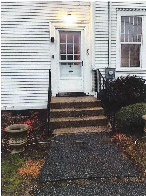
Figure 1 South entry has steps making it inaccessible
