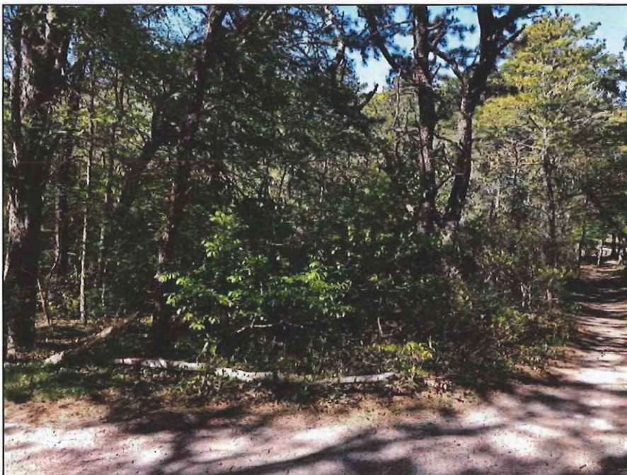
Photo No. 14.: Downstream slope viewed from left abutment. Note the heavy vegetation.
