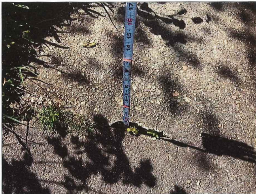
Photo No. 16.: Void within concrete headwall 3 inches deep.
