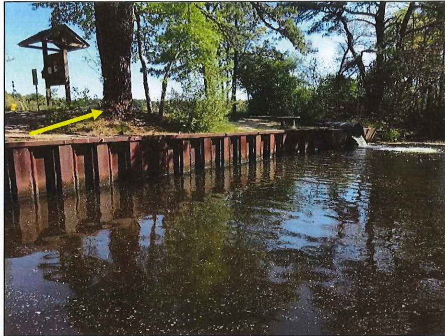
Photo No. 11.: The downstream steel sheet pile wall between the fish ladder and primary spillway outlet. Note 2-foot-diameter tree on downstream side of embankment.
