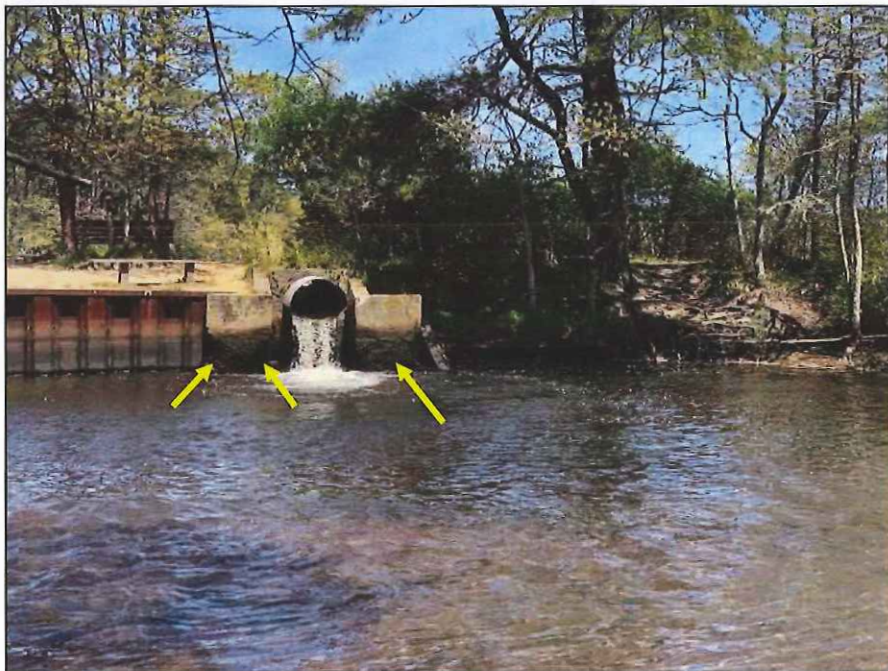
Photo No. 18.: Discharge headwall. Note the scour on the headwall both left and right of the outlet.
