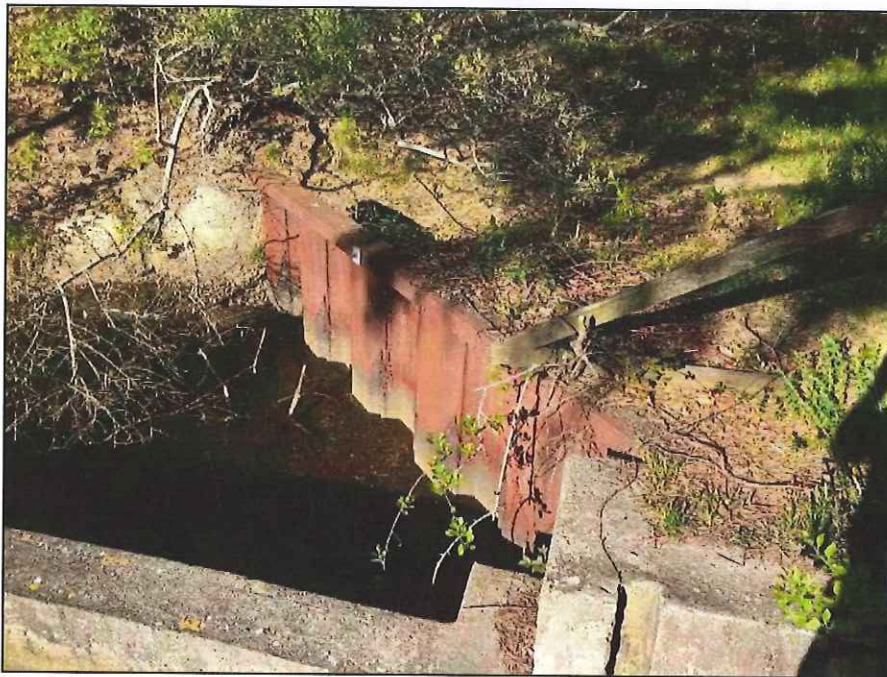
Photo No. 10.: The steel sheet pile wall right of the fish ladder viewed from the fish ladder.
