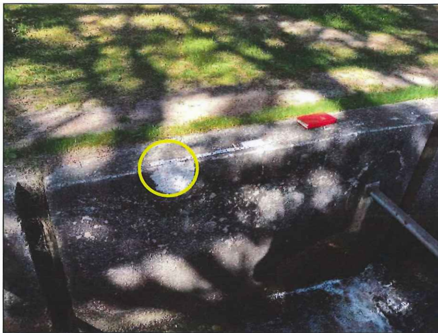
Photo No. 22.: Chip observed on fish ladder downstream of bridge.
