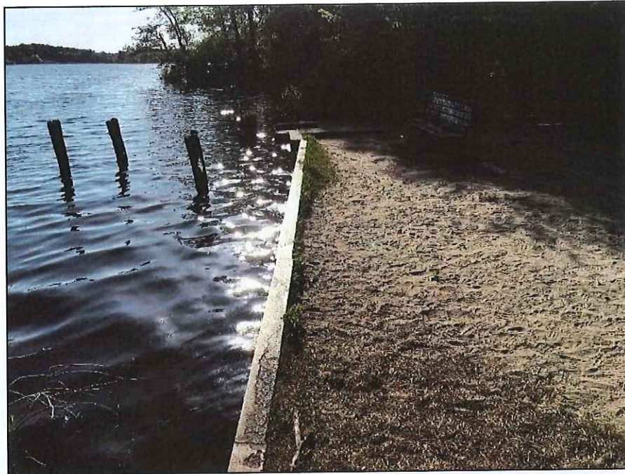
Photo No. 3.: Upstream steel sheet pile wall looking left from near the right end of the wall.
