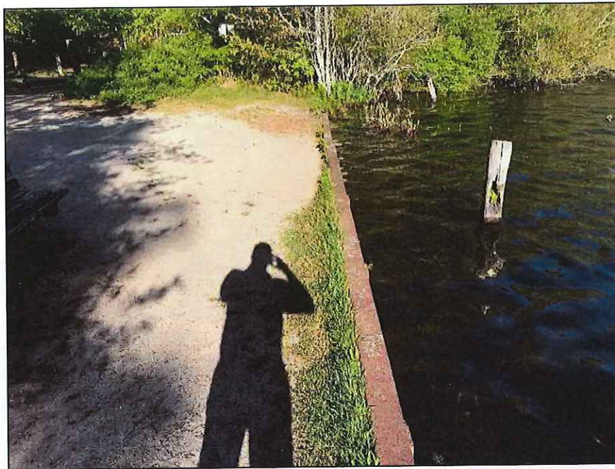
Photo No. 4.: Upstream steel sheet pile wall looking right from the right side of the concrete headwall.
