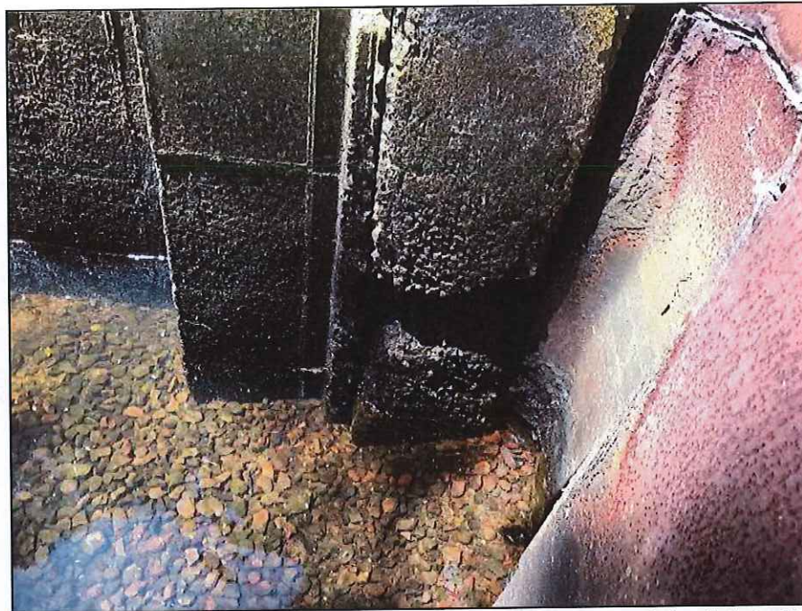
Photo No. 24.: Scour observed at the downstream face of the fish ladder concrete wall adjacent to steel sheet pile wall.
