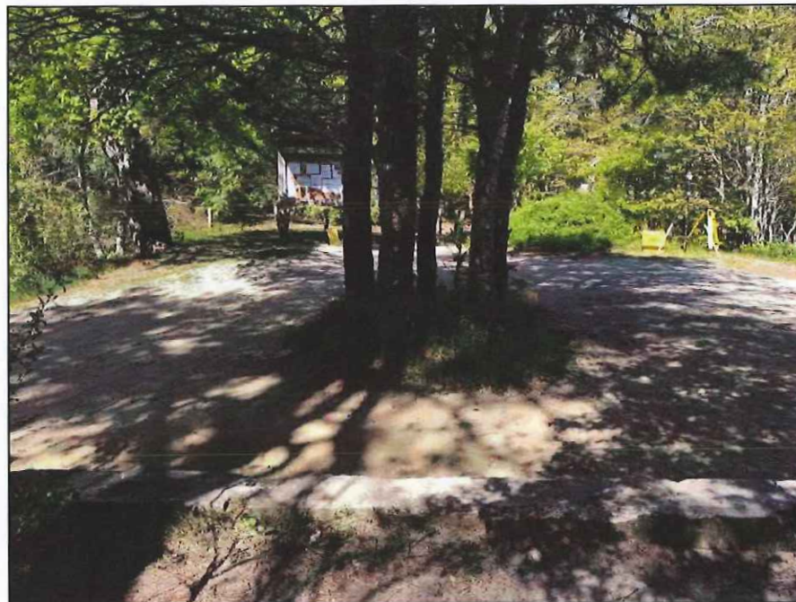
Photo No. 6.: Embankment crest from near STA 1+00 looking right. Note cluster of trees in center of embankment.
