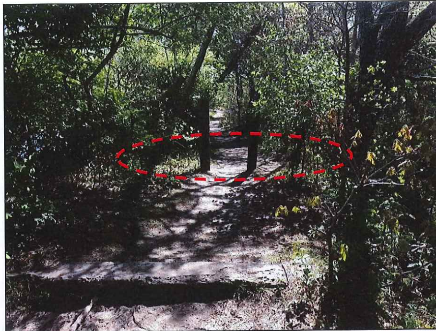
Photo No. 7.: Embankment crest left of the spillway looking left. Note area of apparent past overtopping
