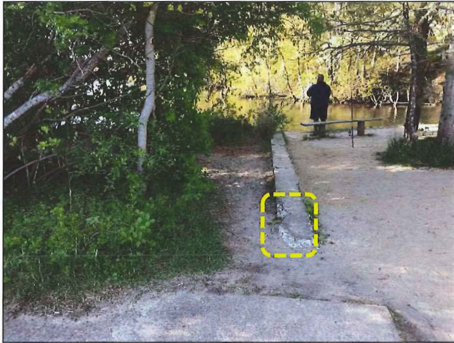
Photo No. 17.: Alignment of concrete intake pipe looking downstream. Note the spalling in the exposed walls.
