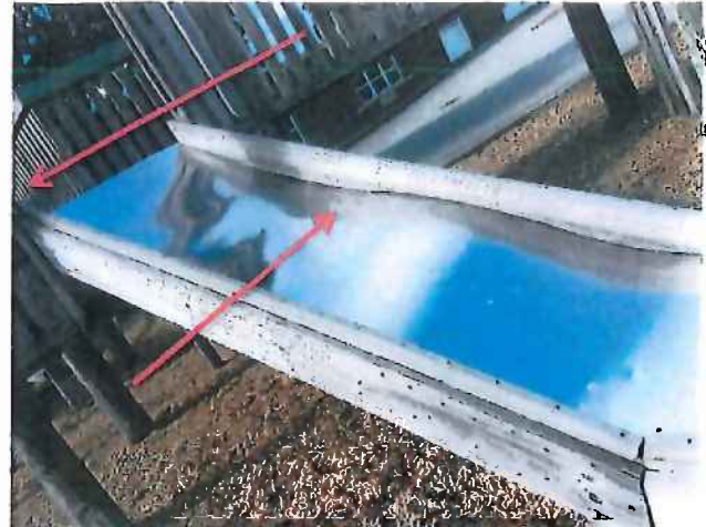
HARDWARE IS EXPOSED. ENTANGLEMENT HAZARD.
