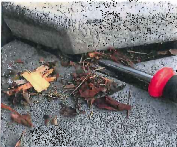
HARDWARE HAS WORN OUT: COMPOSITE PIECE IS TRIPPING HAZARD.
