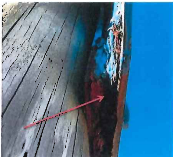
LAYERS OF RUST AND PEEL.
