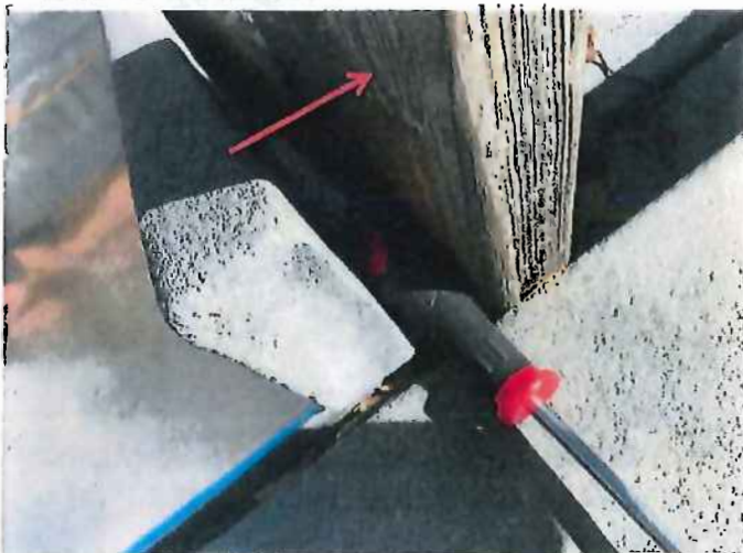
COMPOSITE – WOOD SUPPORT. SEPARATION IS OCCURRING.
