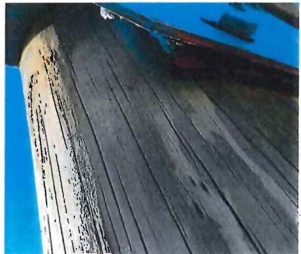
LAYERED AND FLAKING RUST.
