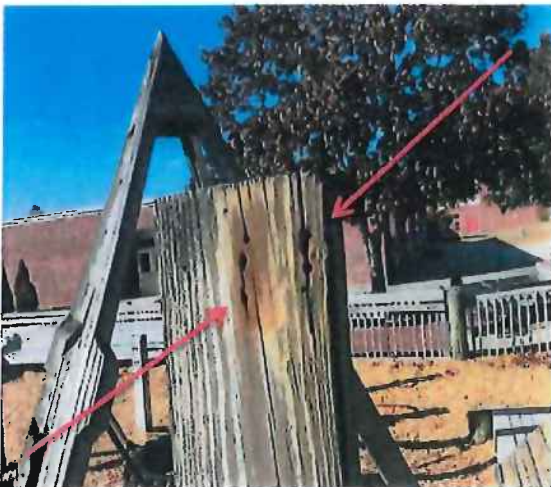
MISSING COMPONENT AND HARDWARE.
