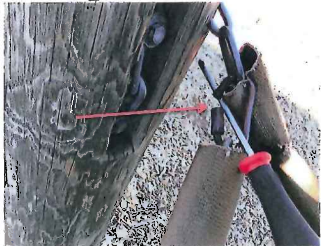
HARDWARE HAS SNAPPED OPEN. INTEGRITY HAS BEEN COMPROMISED.
