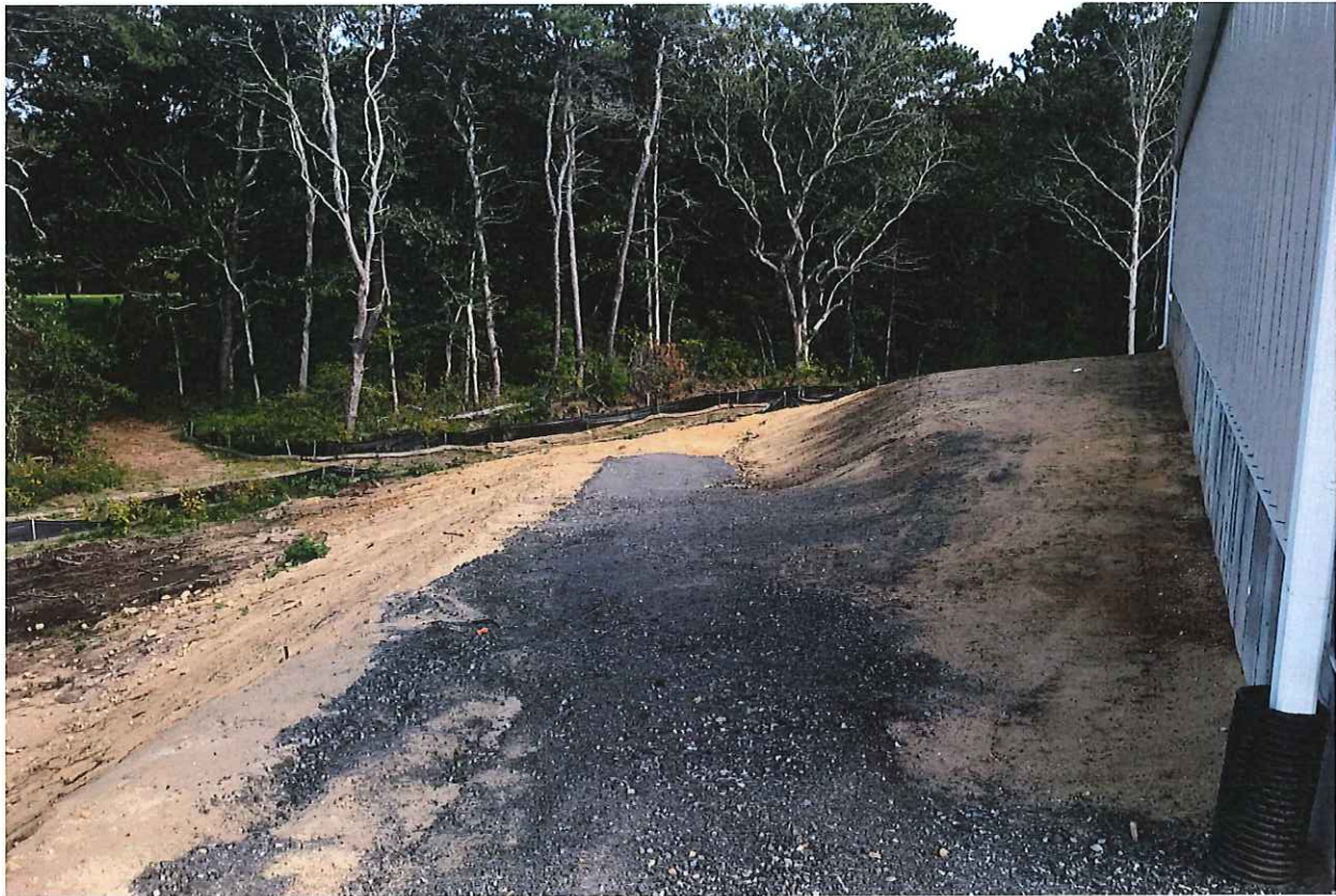
Rough-in of new access road for cart return behind new building eliminating traffic congestion around club house
