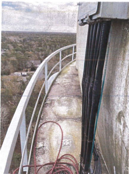
13) Clockwise view of balcony with mildew staining
