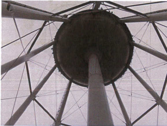
8) Wide view of lower tank bowl with moderate rust staining
