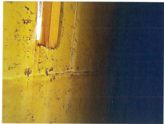
23) Edge corrosion has started at bottom of stiffener beam 4:46
