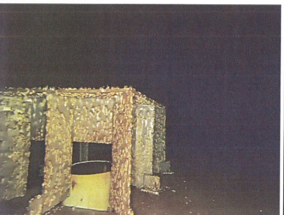
21) Outlet pipe with sediment ring and diffuser 13:11
