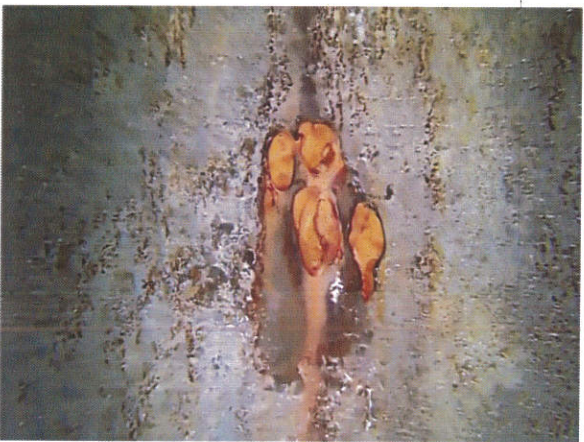
20) Close up of corrosion cells on shell 11:17
