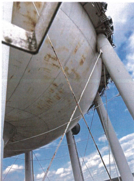
16) View of bowl underside with some surface rust
