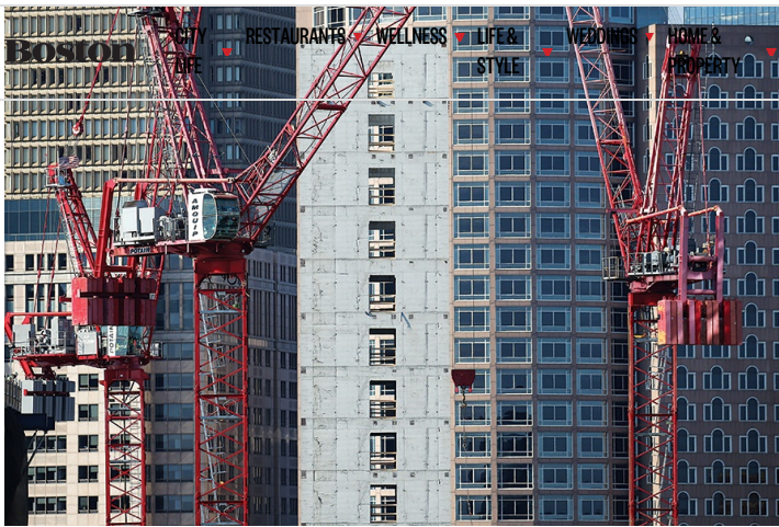
A bird's-eye view of construction in the Seaport District. / Photo courtesy of the Boston Globe via Getty Images
