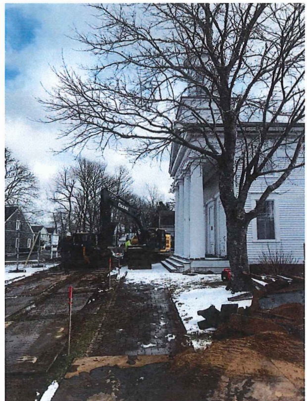
Figure 2 North entry has steps making it inaccessible
