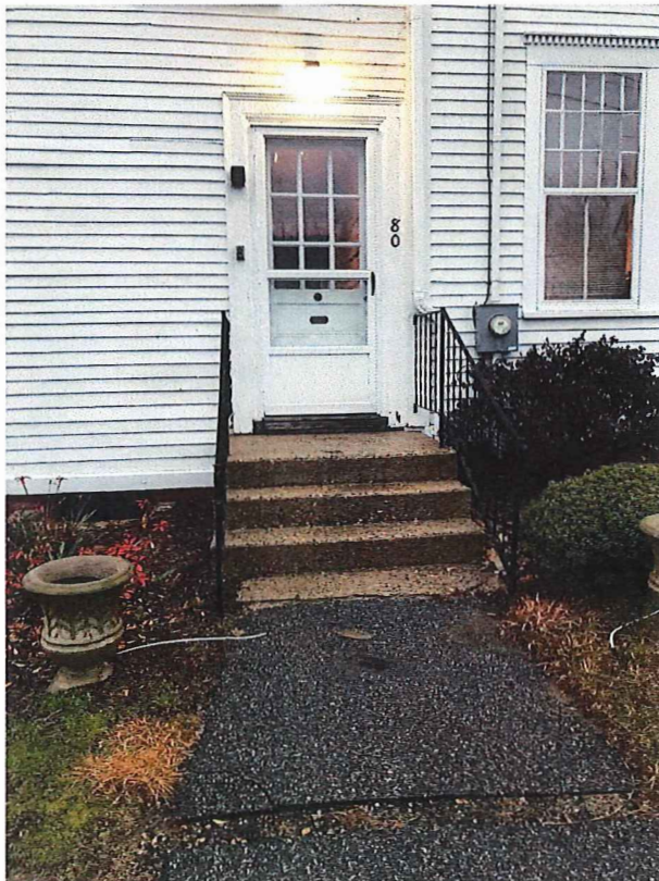
Figure 1 South entry has steps making it inaccessible
