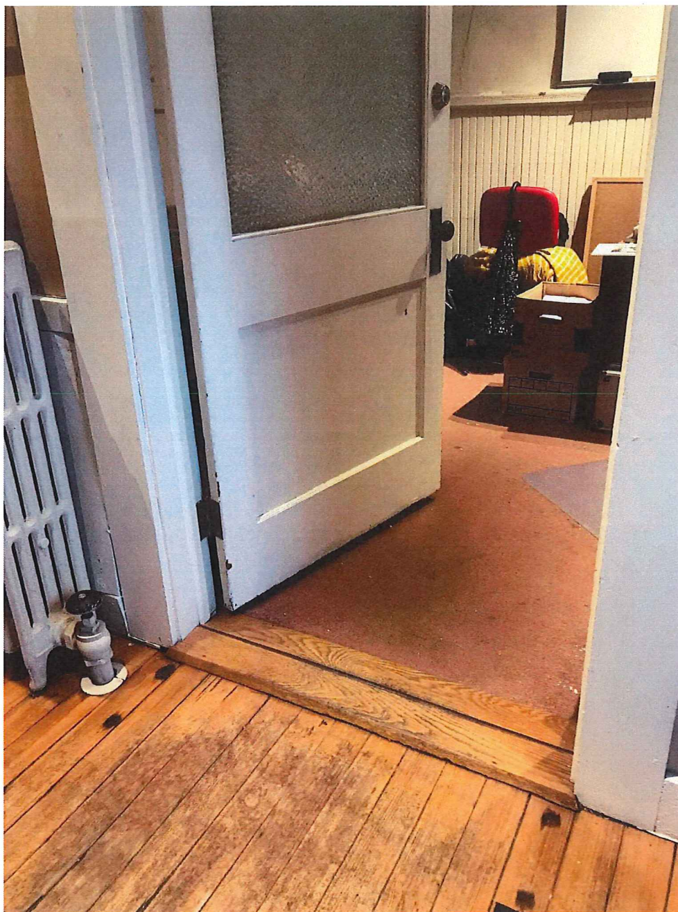
Figure 3 Most interior doors have inaccessible thresholds and hardware
